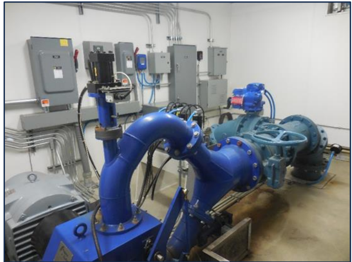
Hydroelectric turbine in Frostburg, MD. Photo courtesy of the City of Frostburg.
