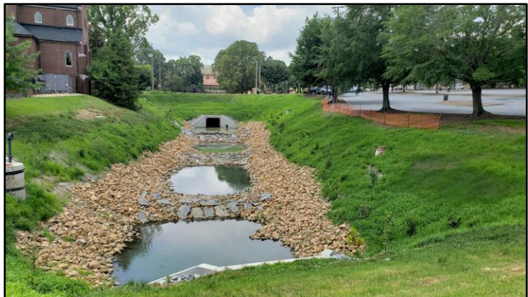
Greenville Regenerative Stormwater Conveyance. Image courtesy of WK Dickson.
